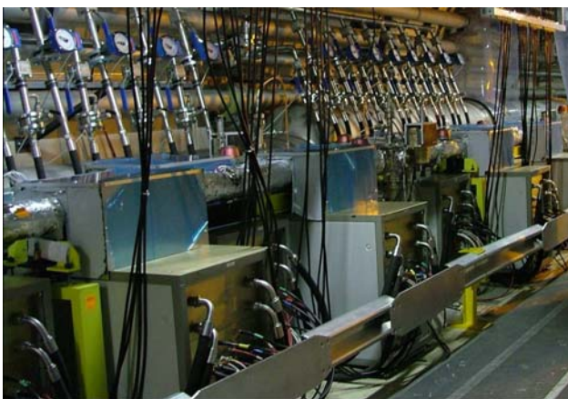
Fig. 1. Kickers and amplifiers in the LHC tunnel
