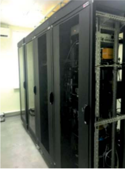
Fig. 2. Example of the racks for the Slow Control electronic equipment
