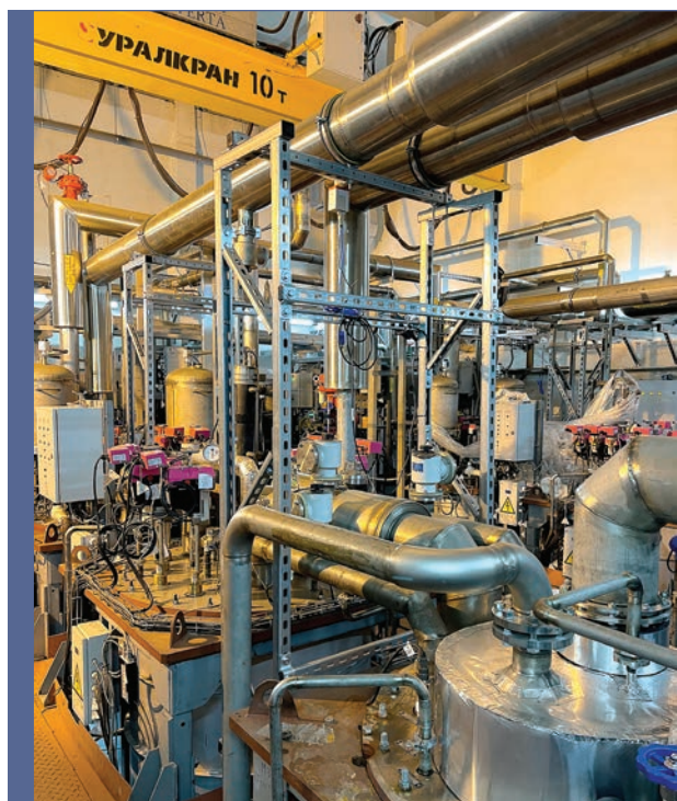
The helium satellite refrigerators RSG-2000/4.5 Nos. 2 and 3 of the Collider
