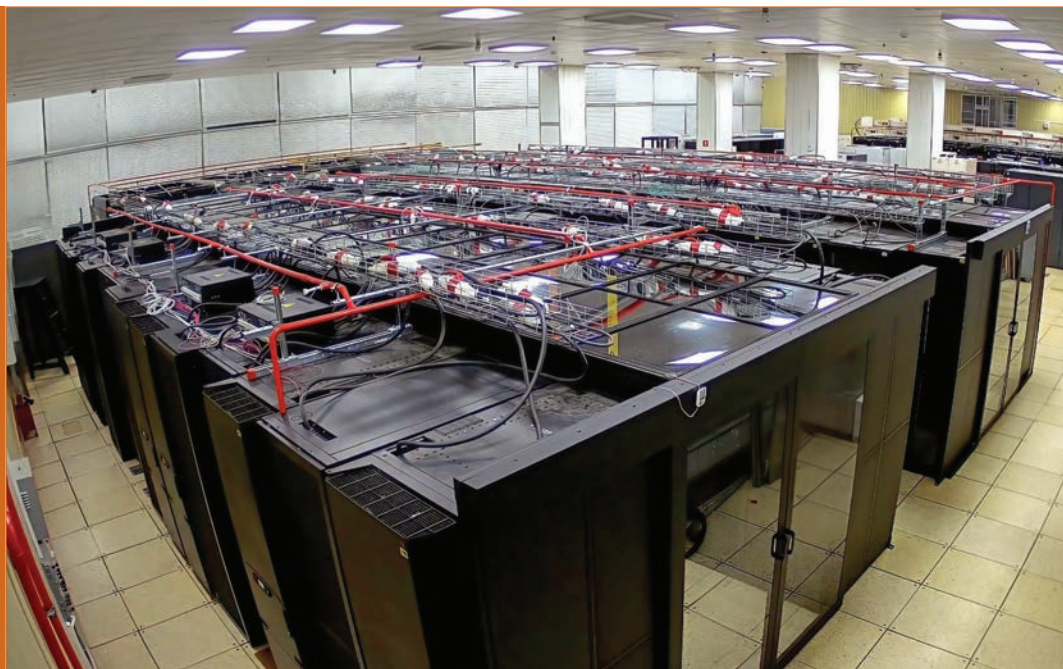
Top view of upgraded Modules 1 and 2, transferred to the cold corridor cooling with inter-row air conditioners, in the MICC machine hall
